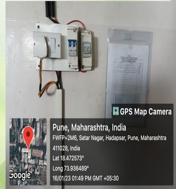
Electric supply through solar energy
