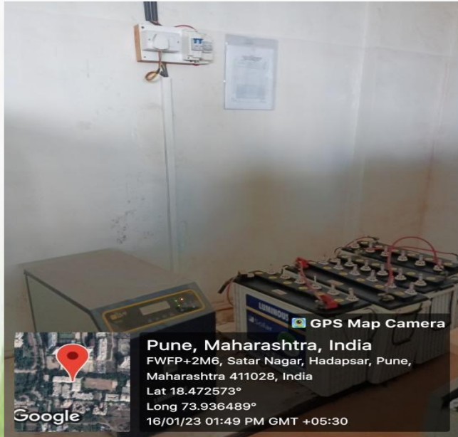
Solar to battery connection for electric supply
